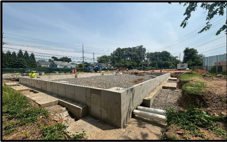
Waterline Piping Entering the Building
