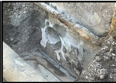
8" diameter open to extend clean water pipe to fair lawn air stripper treatment building.
