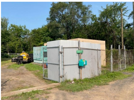
The foam boards around the fence near the generator that will help reduce noise during operations.
