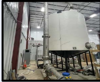
Incoming Water Piping
