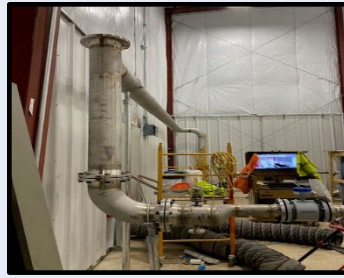
Outgoing Water Piping
