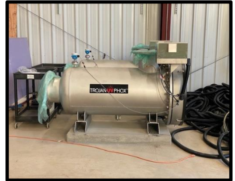
Ultraviolet Oxidation Units
