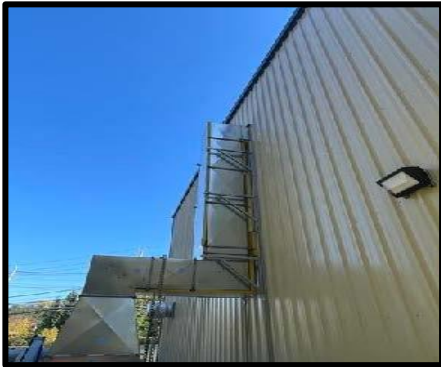
Heating Unit Air Duct
