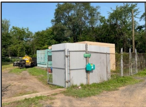
Foam boards to reduce noise from generator
