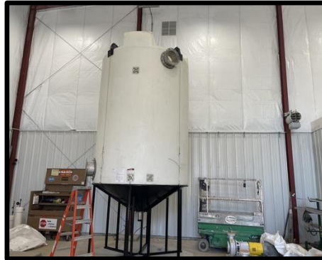
Groundwater Holding Tank
