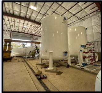
LGAC Set in the Building
