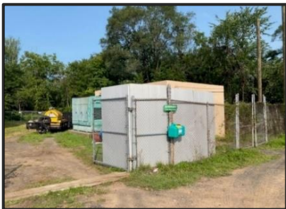
Foam boards to reduce noise from generator
