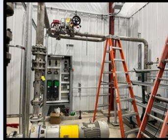
Control Panel Wiring
