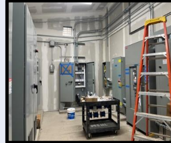
Control Panel Wiring
