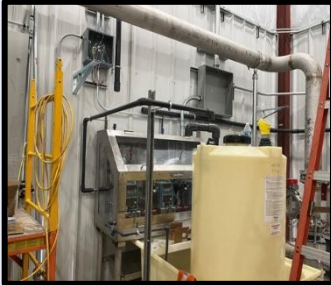
Chemical Feed Pump
