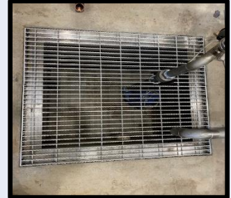
Floor Drain and Pump
