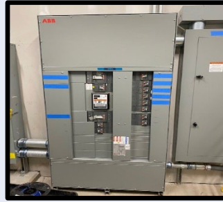
Electrical Control Panel
