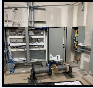
Control Panel Wiring
