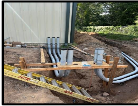
Electrical Service at Treatment Building
