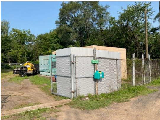
The foam boards around the fence near the generator that will help reduce noise during operations.
