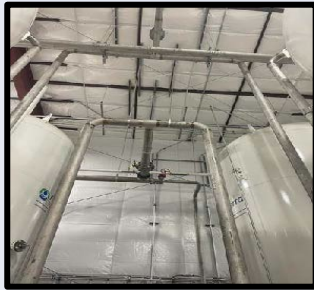
Pipes Between Carbon Units
