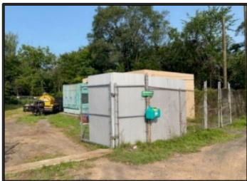
Foam boards to reduce noise from the generator.
