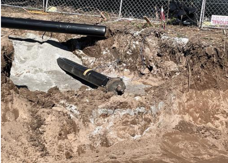
Water Line Pipes at the New Treatment Building
