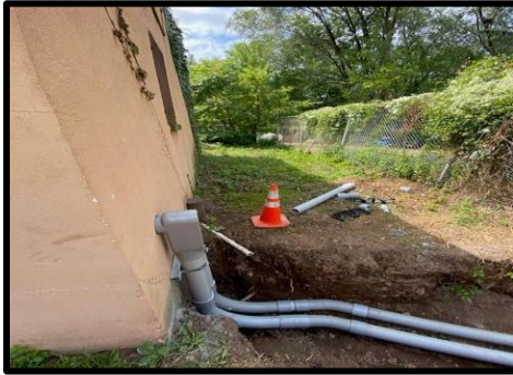
Electrical Conduit Connection to Fair Lawn Building
