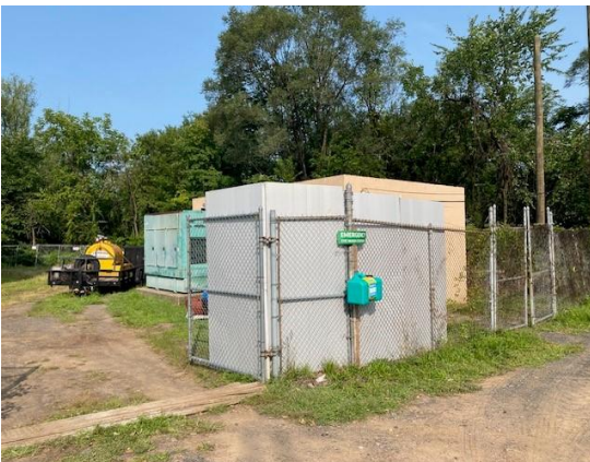
The foam boards around the fence near the generator that will help reduce noise during operations.
